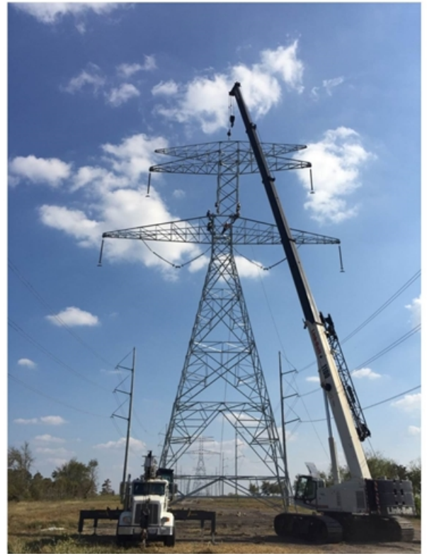
Construction of a new permanent 345kV double circuit tower in between temporary bypasses to safely reenergize circuits damaged by tornadoes in April 2015.
