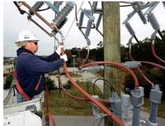
A Houston Electric lineman working on lines damaged by storm the week of April 17 th
