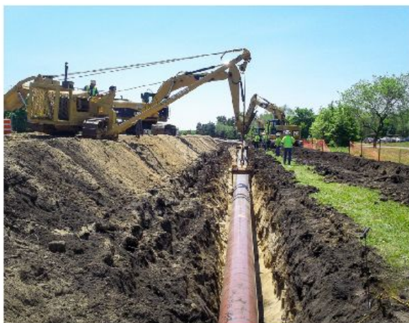
One of many modernization construction projects, Belt Line is scheduled to be completed in 2023.
