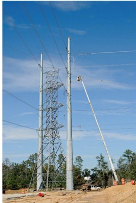
Raising our high voltage transmission towers to accommodate the new Highway US-99 corridor and to serve load growth
