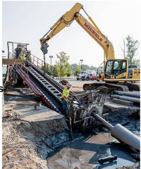
Using horizontal directional drilling to construct and install a new pipeline under the bed of the Arkansas River
