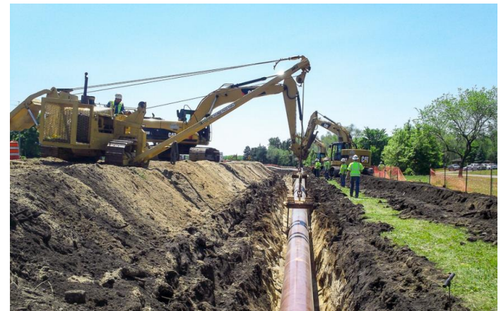
Work on the beltline project in MN – Infrastructure Services completing work for Natural Gas Distribution
