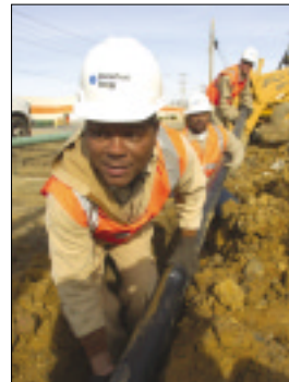
FRONT TO BACK, WILLIE LEWIS, FIELD ESTIMATOR, TONY JACOBS, TECHNICIAN, AND JIM BRUSH, LEAD TECHNICIAN, LAY REPLACEMENT PIPE IN LITTLE ROCK, ARKANSAS.
