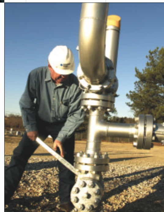
TECHNICIAN JERRY MATHEWS MAKES SURE BOLTS ARE TIGHT AT THE PERLA STATION.
